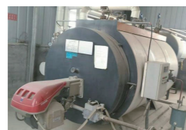
■ Air supply fan for boiler
