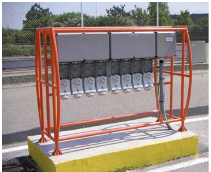
Container Terminal, Le Havre – France
